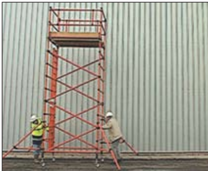
Diagram showing tower being moved, clearance of 25mm on stabilisers and maximum platform height when moving of 4.0m.
